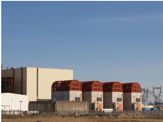
3-MWe station blackout diesel generators [DUS]
